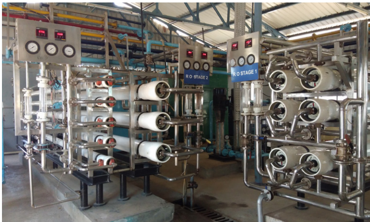
Advanced three-stage water treatment plant for water recycling
